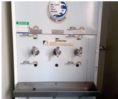
Water Filtration System : Ensures access to safe and purified drinking water, maintaining hygiene and well-being across the campus.
