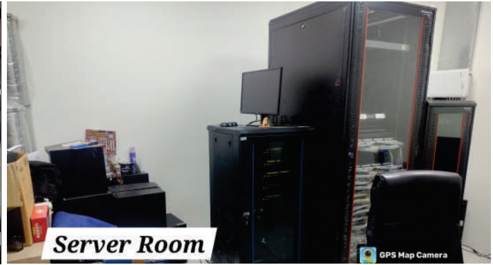
A dedicated facility ensuring secure data storage, seamless connectivity, and efficient management of the college's digital operations.
