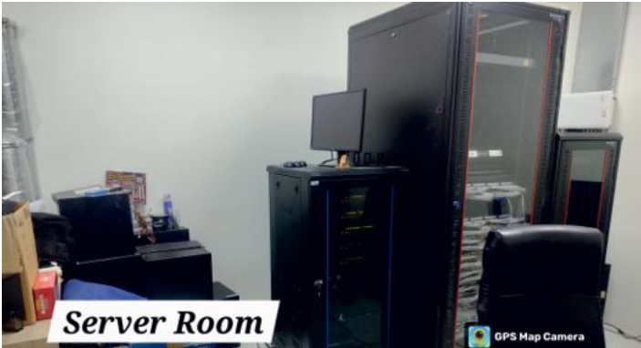
A dedicated facility ensuring secure data storage, seamless connectivity, and efficient management of the college's digital operations.
