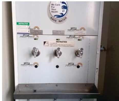
Water Filtration System : Ensures access to safe and purified drinking water, maintaining hygiene and well-being across the campus.
